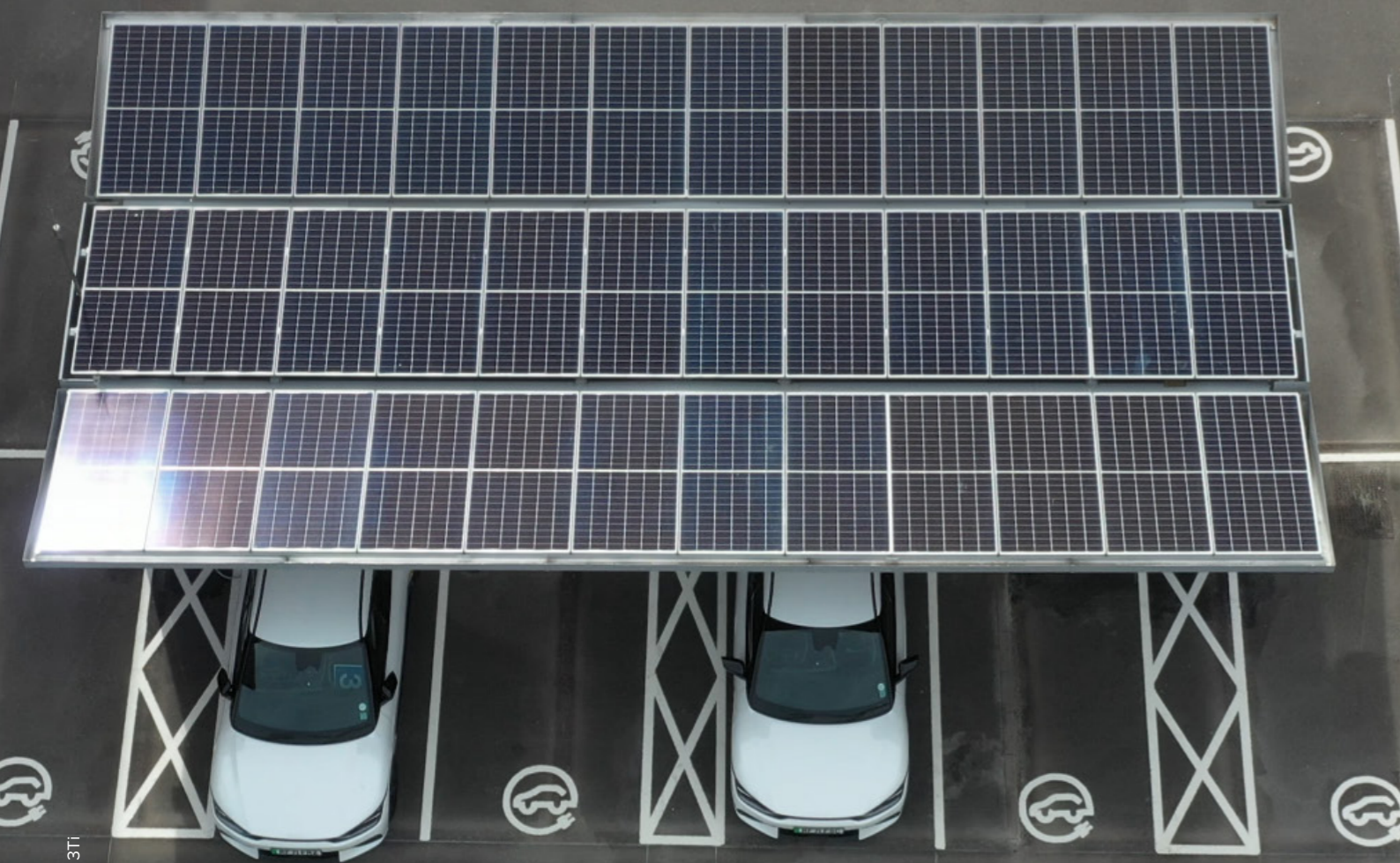
3ti 'Papilio3' Pop-up Solar Car Park installed at SRP
